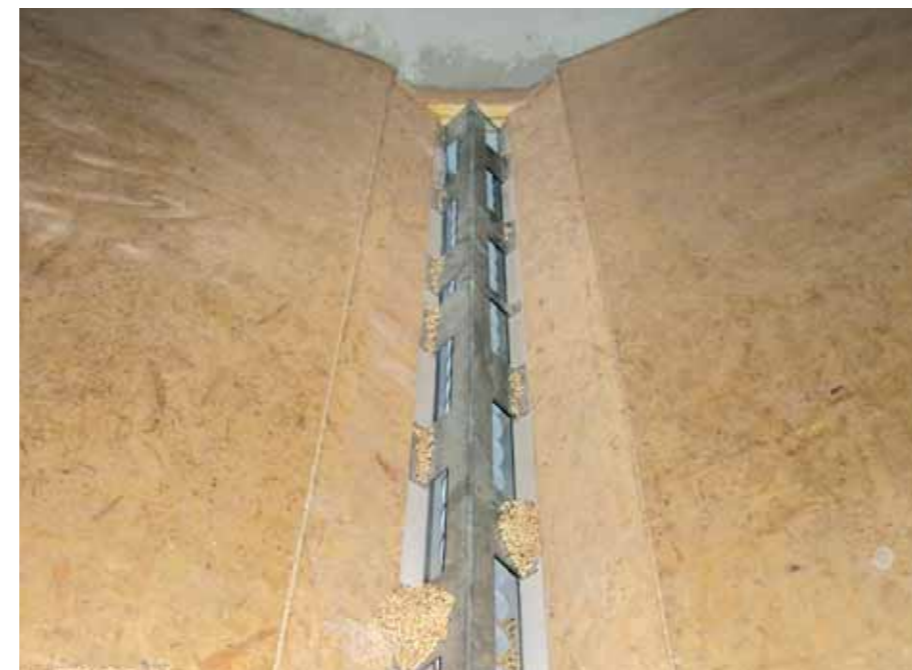
The HDG pellet delivery worm conveys pellets from rectangular storage rooms.
